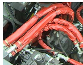
Fire resistant sleeves on hoses
